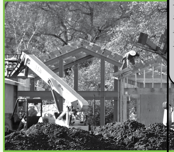
Construction continues on Hanna's new facilities, including the 7,800-square-foot Admissions and Alumni Center and 8,950-square-foot Multi-Use Auditorium.
